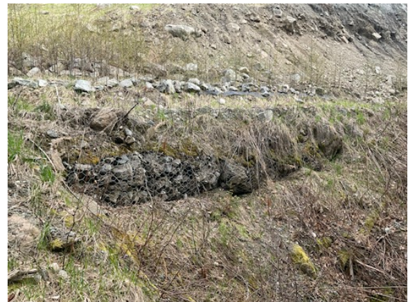
Erosion at base
